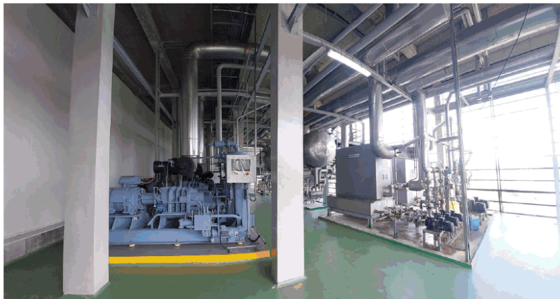
The BoxFreezer's machine room accommodates a compact and energy-efficient freezing unit for the plant.
